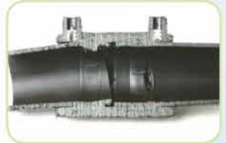
Off-Centering of the Pipe on the Left Side and Wrong Welding Parameters Setting
